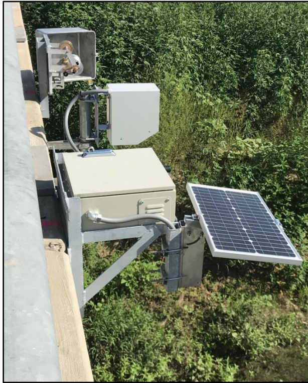
Figure 2.2 Image of a completed RQ-30 gauge installation. Photograph by Scott Grzyb, U.S. Geological Survey.
